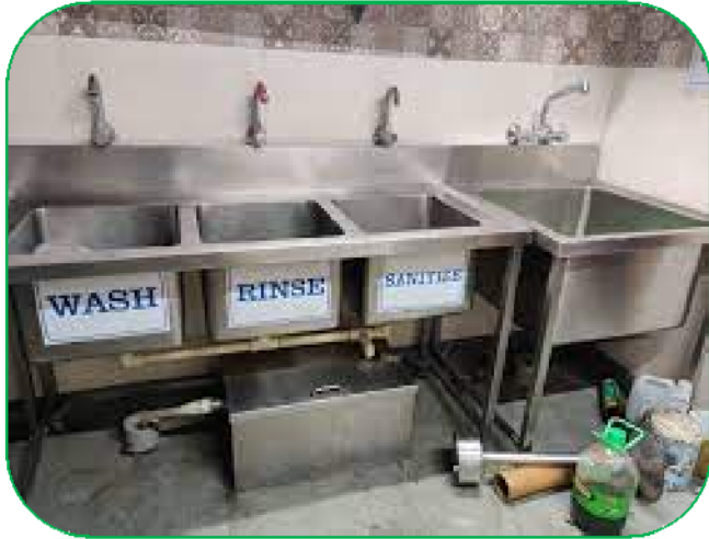
3 UNIT S.S SINK
